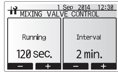
Mixing valve control setting screen
